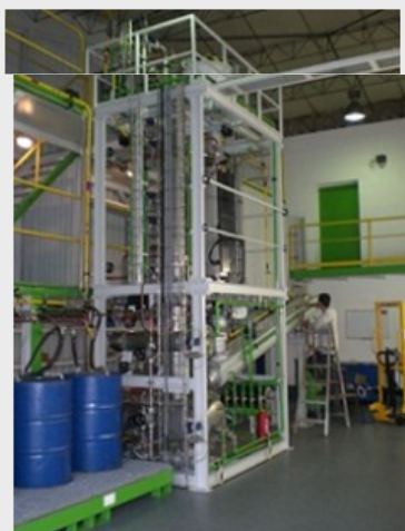
Pyrum Innovations, a German/French startup working on a newly invented recycling process for used tyres, is one of a growing numbers of cleantech companies that have joined the Autodesk Clean Tech Partner Programme.
